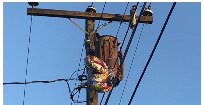
When foil balloons (plastic covered with metallic paint) contact power lines, they cause thousands of customers to lose power. Photo by Katie Register, CVW.
